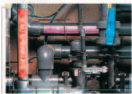
Identify pipelines on-site!
